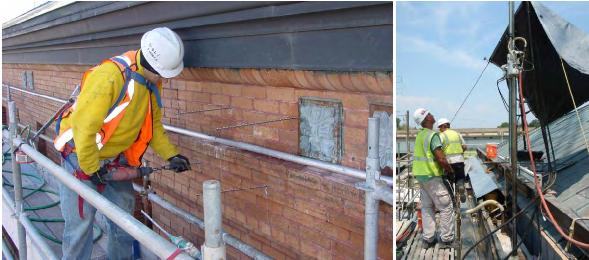
Fig. 6 At left, installation of helical wall ties into existing clay brick masonry walls. At right, coring at the top of the exterior walls in order to insert vertical reinforcing.
