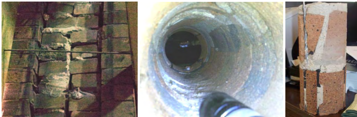
Fig. 10 Left, view of voids in brick masonry prior to injection at window jamb. Middle, view looking into a core hole made after completion of CIF injection showing the lighter colored CIF material has filled the voids in the wall. Right, core extracted from the exterior wall by the electrician after completion of CIF injection showing a helical wall tie and filled voids.
