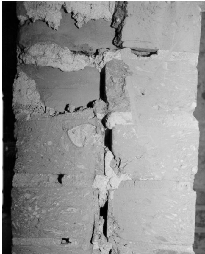
Figure 2. Typical section through interior shear walls, showing many internal voids and incompletely filled mortar joints. Interior voids were channeling water from gutter and roof leaks throughout the wall, resulting in mortar deterioration and related freezing damage.
